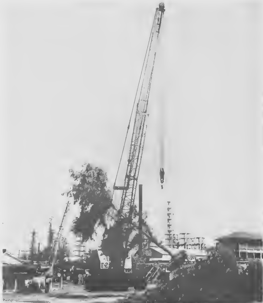
WITH a grinding wrench, a derrick was busy earlier this month ripping out trees in front of the old Esso Dining Hall. The dining hall was also torn out to make way for a parking area and new colony by-pass road.
